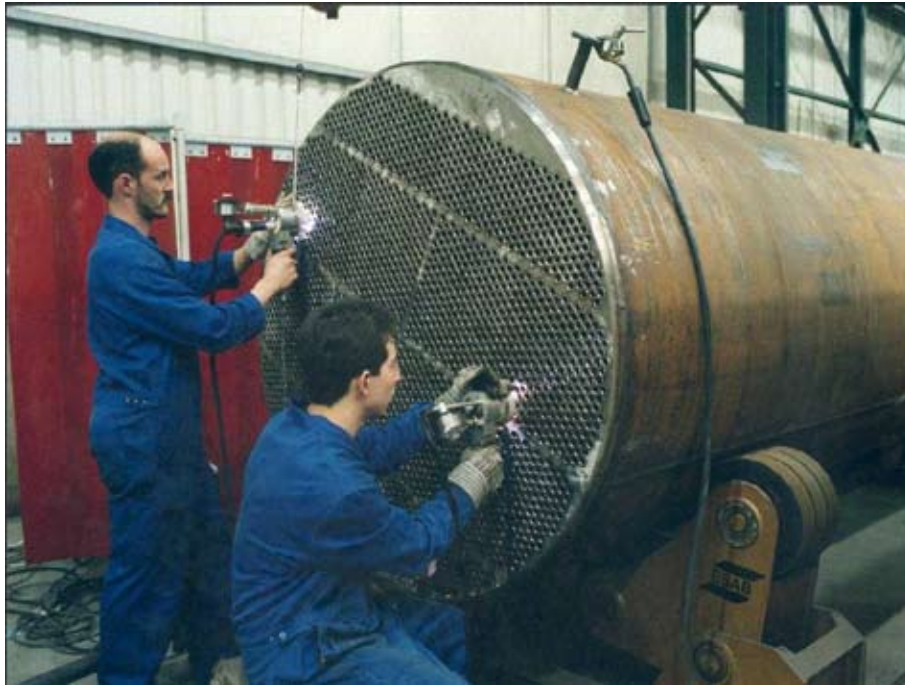
FIGURE 10. Condenser in Zeron 100 for a VCM plant
