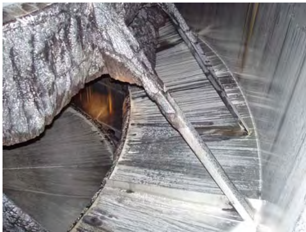
Figure 20: N80367 liquid distribution rings at NIPSCO Schahfer Station.
