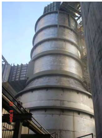
Figure 12: Absorber tower at Santee Cooper Winyah Station.
