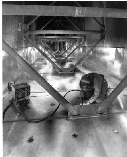
Figure 13: IP&L Flue Gas Duct with N08367 Alloy Lining
