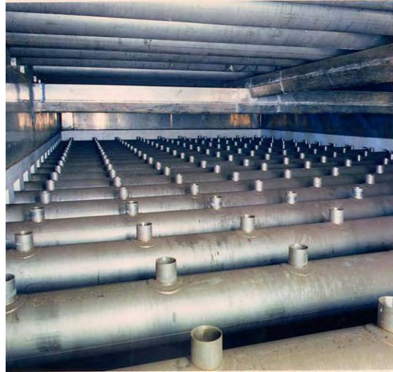
Figure 6: N08367 Alloy Spray Piping
