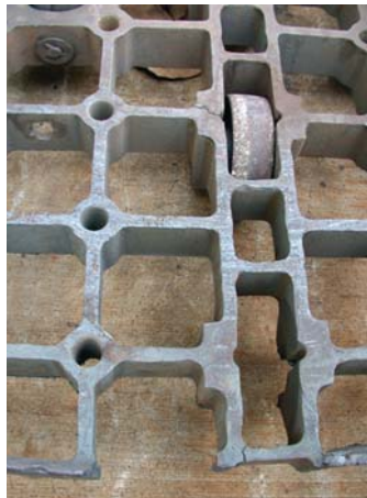
Fig. 3. Close-up of cast tray after 18 months service prior to weld repair to replace lost segments due to fracture from thermal cycling
