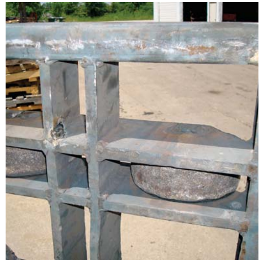
Fig. 4. Wrought fabricated tray photo taken after five years in service.
